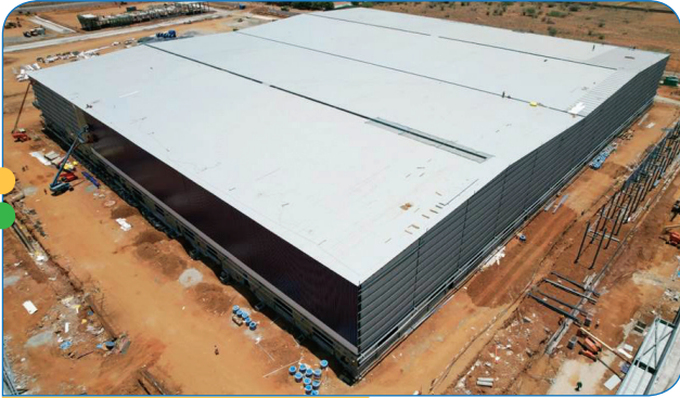
TP Solar Limited, Tirunelveli
